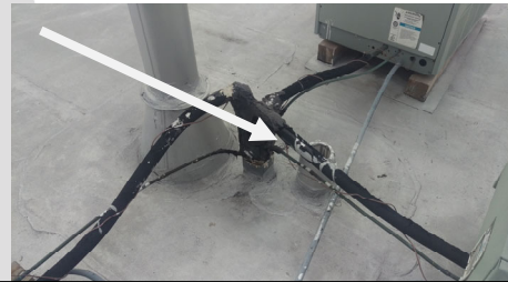
Damaged/missing insulation at A/C lines
