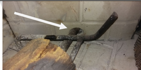
Gaps where gas line enters fireplace
