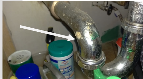
Corroding metal drain pipes
